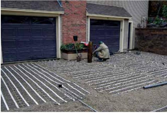
Figure 10. Electric heat tape snow melt system is installed in the bedding layer of permeable interlocking concrete pavement.
